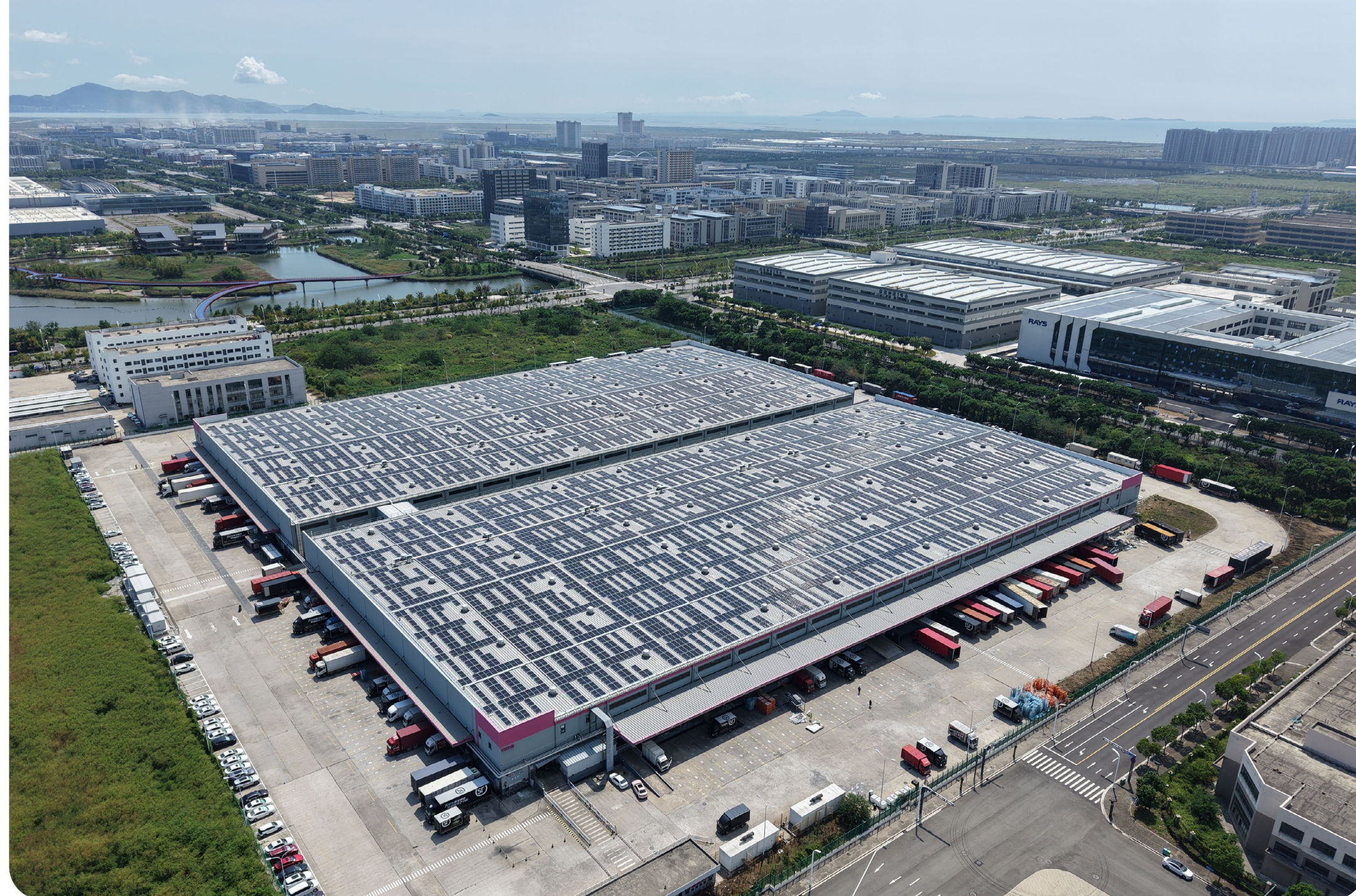
▲ Rooftop photovoltaic facility at the Vipshop Wenzhou Bonded Warehouse
